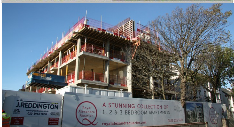
The restored Alex as it will look (top) and work in progress on Dyke Road
